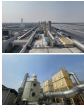
Exhaust Gas Treatment Facilities
